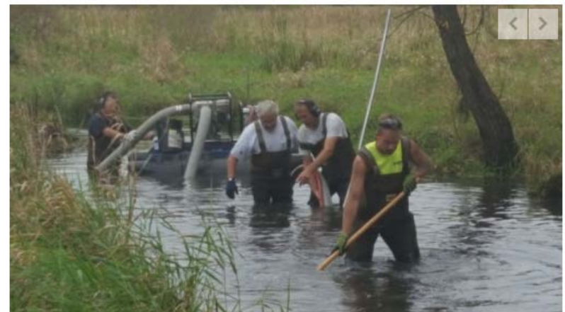
Workers vacuum phosphorus-laden muck from the bottom of Dorn Creek this week.
