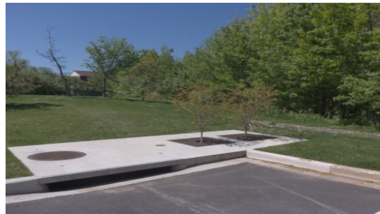
Filterra Sedimentation Chamber
